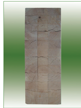
Example of Checking
